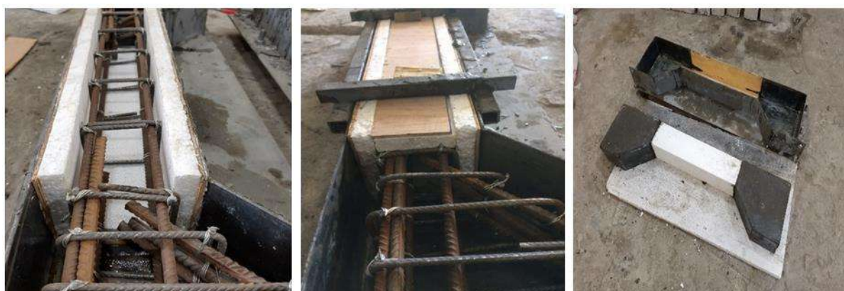
(a) Hybrid section column reinforcement (b) Hybrid section mold and steel reinforcement (c) Hybrid section after casting
